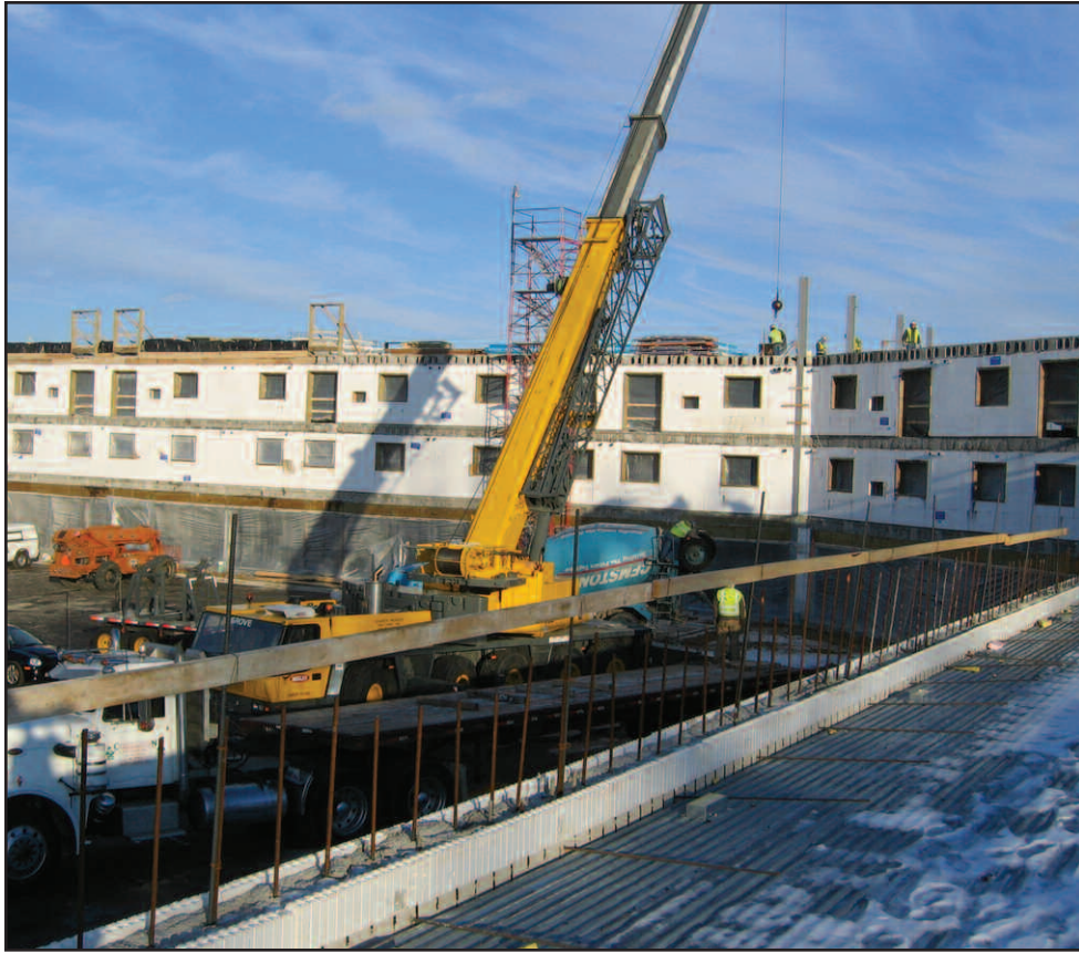
Work is being done in stages on the project with the ICF walls poured and allowed to cure before the hollow core plank is positioned for the floor.
