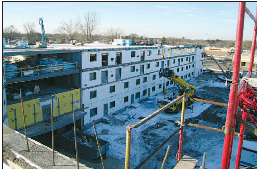
This rooftop view of the Village Plaza ICF project shows crews at work on various levels.
