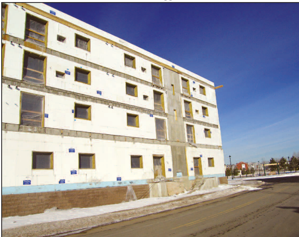
The four-story Village Plaza multi-use facility in Circle Pines is the largest ICF project in the Upper Midwest.
